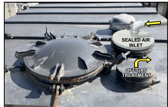
Sealed Flange Air Injection for Off-Gas Treatment
