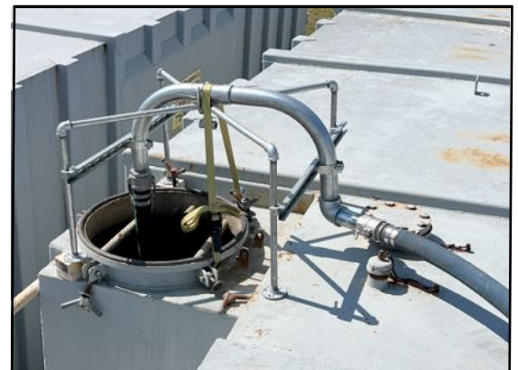
Air Inlet Anti-Siphon Manhole Light Cage Mounted on Frac Tank
