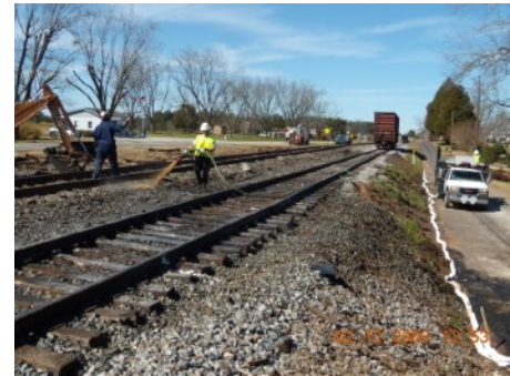
At-Grade Crossing Diesel Release
