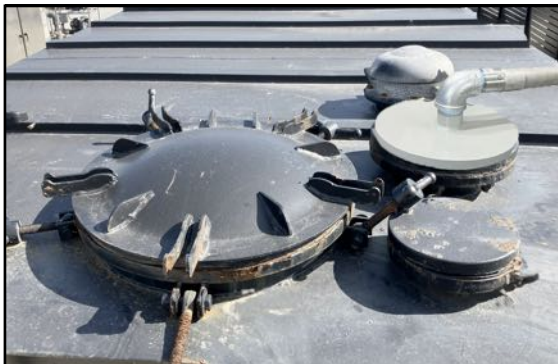
Sealed Flange Air Injection for Carbon Off-Gas Treatment
