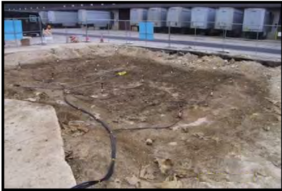
16 Biosparge Points in UST Tank Pit
