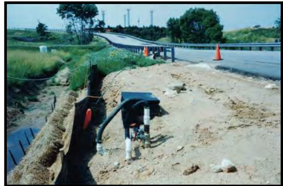
BioVenting System with HC-2000 Injection
