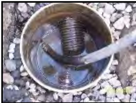
Oil Leachate Collection Sump
