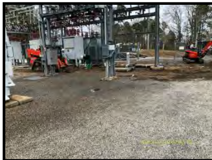
Regulator Explosion at Substation
