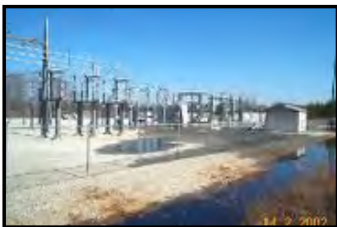
Transformer Oil Release
