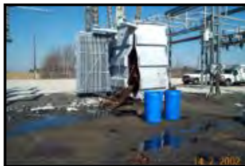
Closeup of Transformer Oil Release
