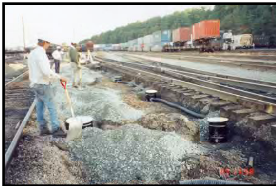
Leachate Perforated Pipe and Sump Collection System
