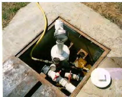
BioFoam Injection Well Head
