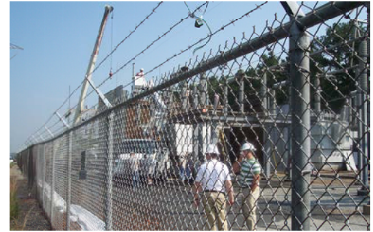
Transformer Explosion at Substation
