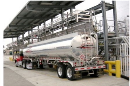
Lubricant Tanker Loading Rack
