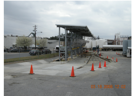
Construction of Secondary Containment Rollover Spill Containment and Clean Stormwater Pavement Diversion Transitions
