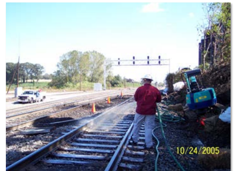
Initial Treatment of Tracks with HC-2000 and Excavation of Saturated Ditch Soils
