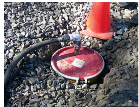
Leachate Collection Sump Between Tracks With Pump Out Stinger
