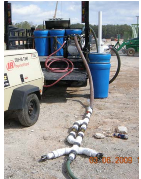
Remtech JetVac Dual Phase Vacuum Extraction System
