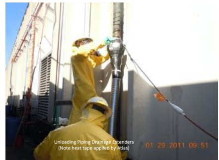
TDI Thawed with Heat Tape, Drum Heaters, and Steam and Drained from System
