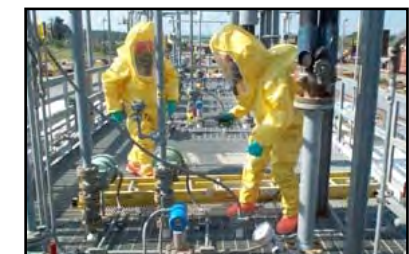
Anhydrous NH 3 Training at Coal Fired Power Plant for NO x Removal
