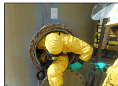
Leaking Sulfuric Acid Tank Cleaning
