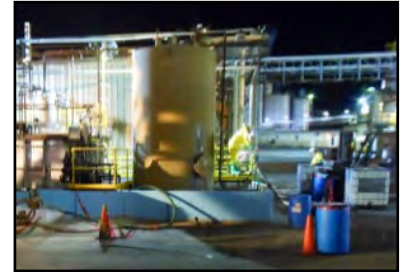
Leaking Sulfuric Acid Tank Transfer
