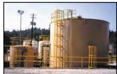
Remtech Groundwater Treatment System at Superfund Site
