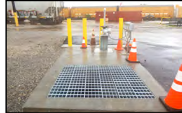
Stormwater Vault Containment, Automated Gate & Hydrocarbon Sensor
