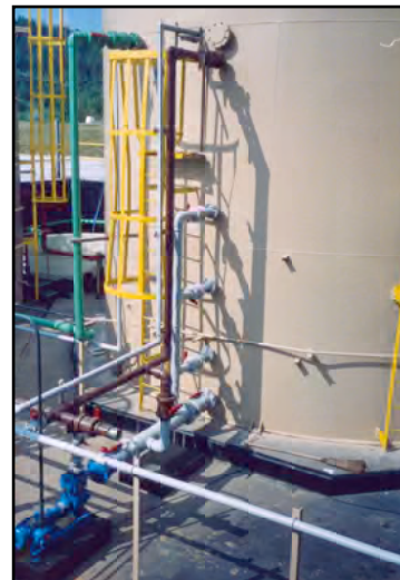
Landfill Leachate Treatment System
