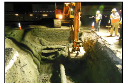
Emergency Response & Remediation at Leaking Fuel Line at Intermodal Yard
