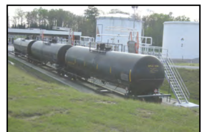
Ethanol Unloading Rack with Secondary Containment
