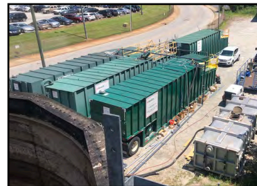
Mobile WWTP Treatment System
