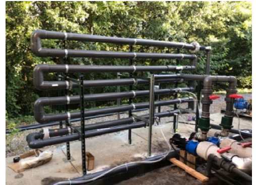
Serpentine Chemical Mixing System Fabricated in One Day for Acid, Base and Alum Addition
