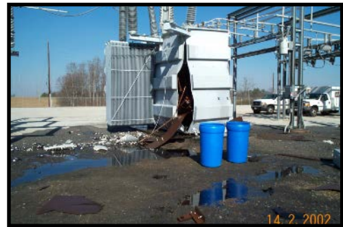
Closeup of Transformer Oil Release
