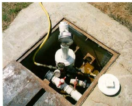
BioFoam Injection Well Head
