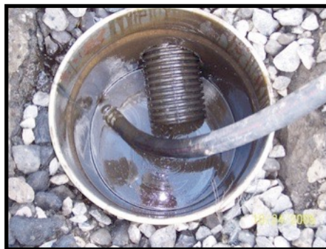
Oil Leachate Collection Sump
