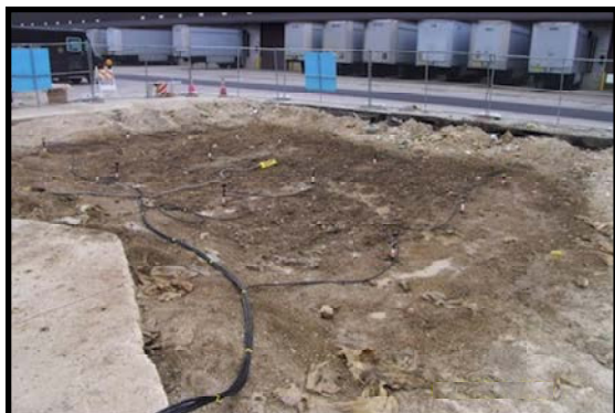
16 Biosparge Points in UST Tank Pit
