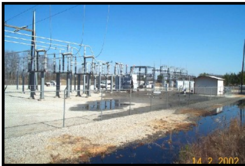
Transformer Oil Release
