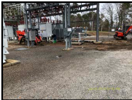
Regulator Explosion at Substation
