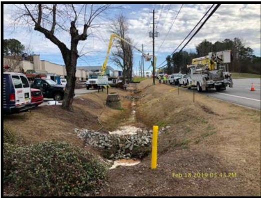
Site Monitored Through Three Additional Rain Events Until Oil Sheen Dissipated in Stormwater Runoff
