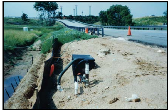
BioVenting System with HC-2000 Injection
